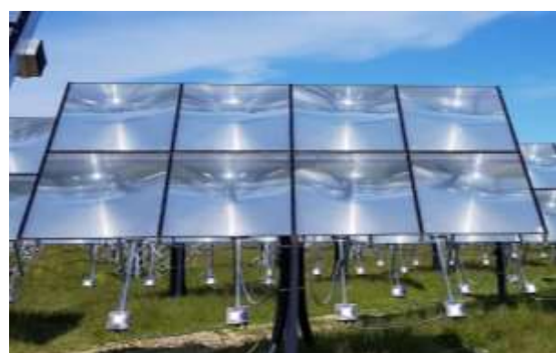
Figure 5: Sun tracking system for the utility scale solar thermal field
